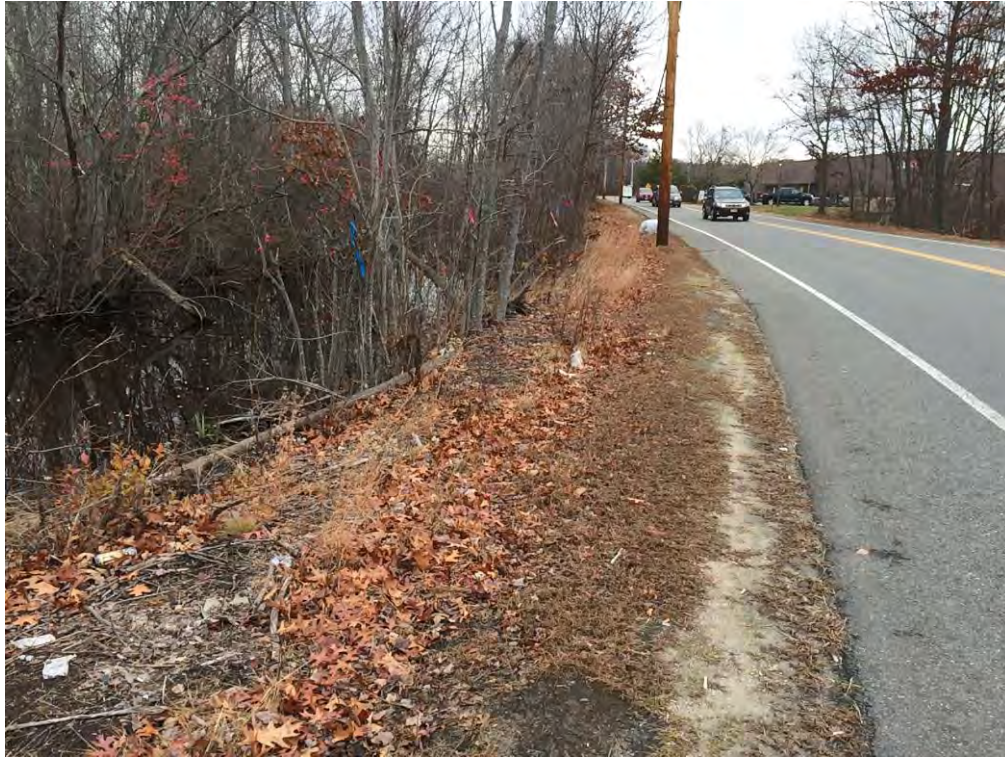
Typical slope along north side of roadway adjacent to wetlands (Sta. 45+00± to 46+00± LT)
