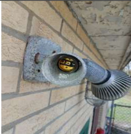
Light gasket debris, not asbestos
