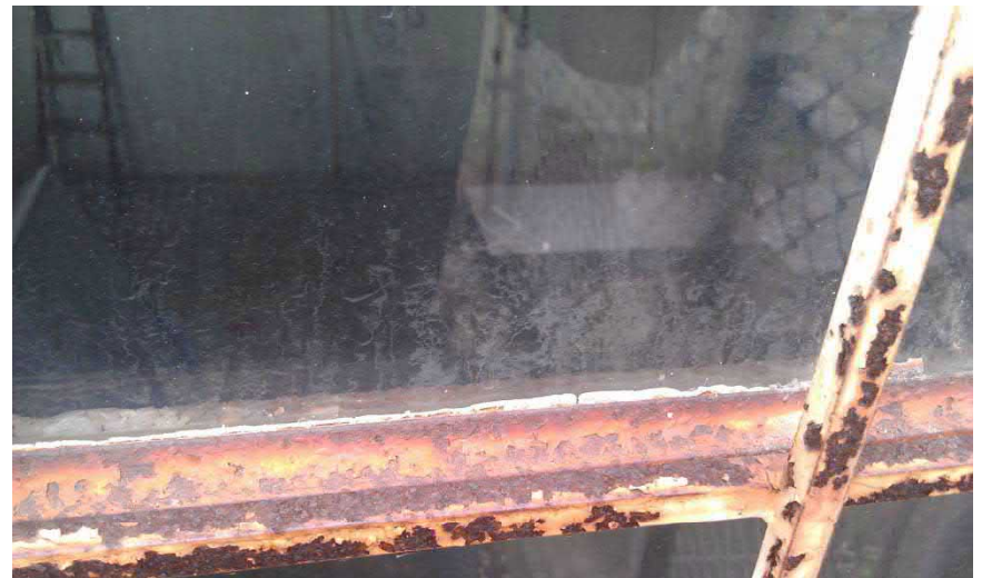
Asbestos Window Glazing
