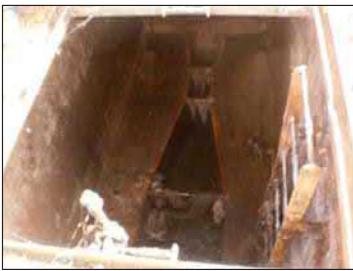
PHOTO 1 PARSHALL FLUME PR-3
