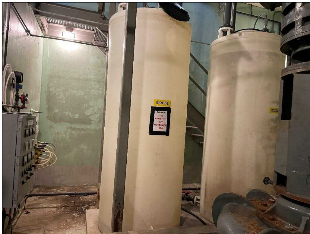
Bioxide storage tanks (foreground), green wall paint and metal staircase (background), lower level
