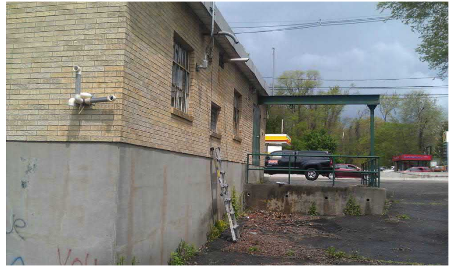
ACM – Window and Louvered Vent Caulking
