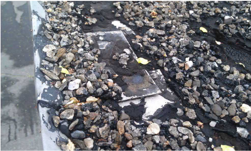
Roofing with Trace Asbestos
