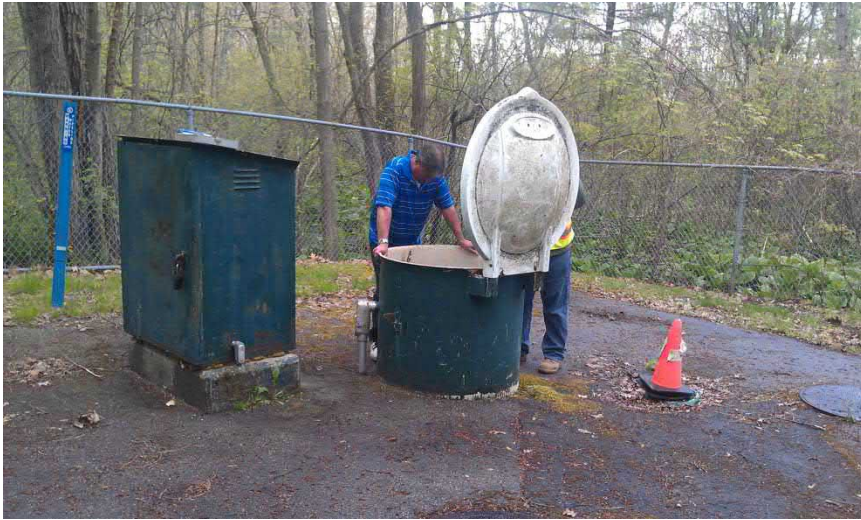
Kittredge Road Pump Station
