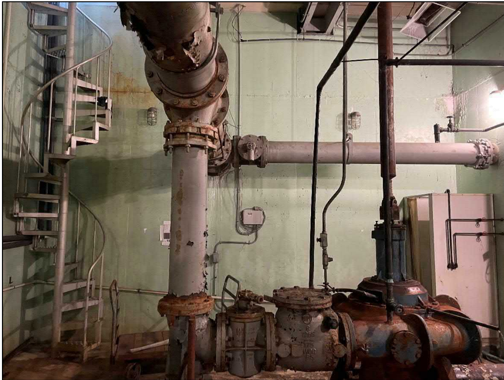
Gray paint on piping and equipment, lower level
