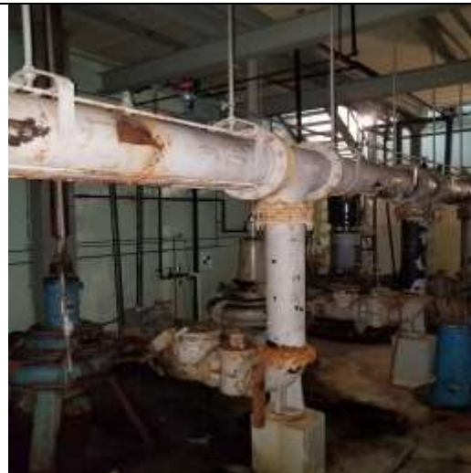
Lower level pipes
