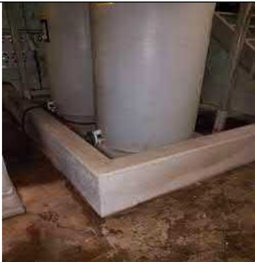
Chemical tank section
