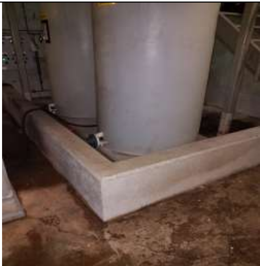
Chemical tank section
