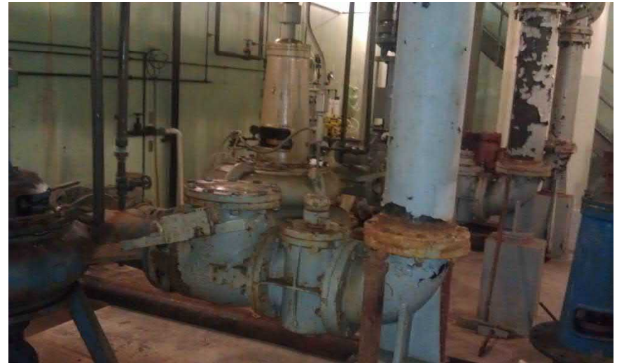
LBP on Basement Pump Equipment
