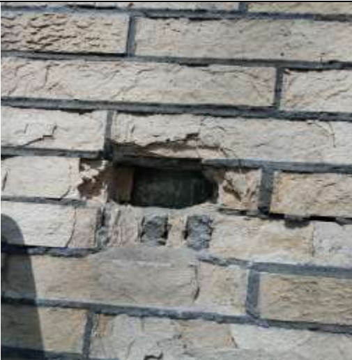
Brick to block wall, no vapor barriers
