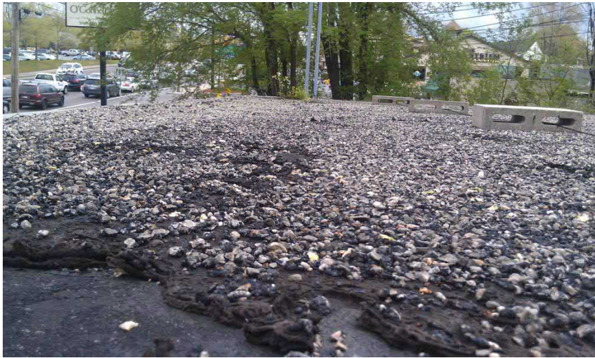
Roofing with Trace Asbestos
