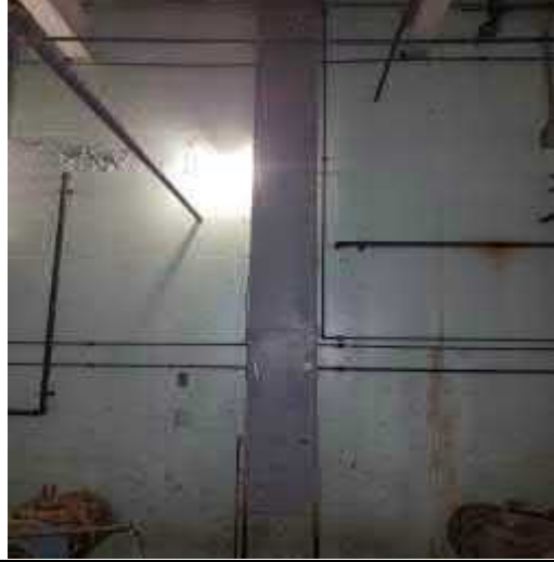
Gray duct paint
