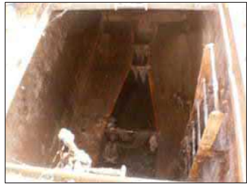
PHOTO 1 PARSHALL FLUME PR-3
