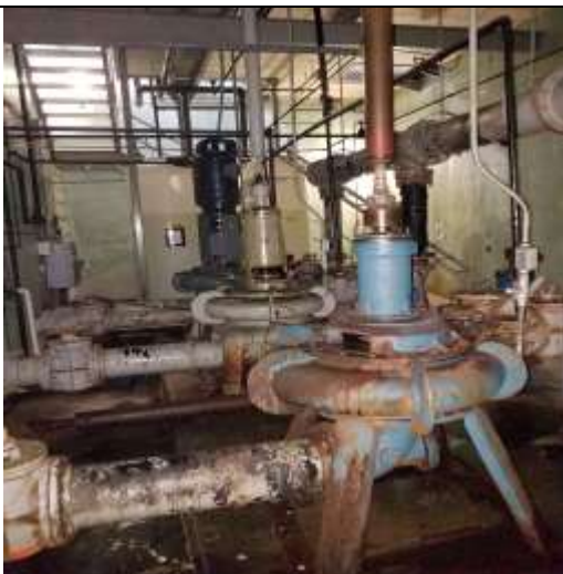
Lower level pipes/motors
