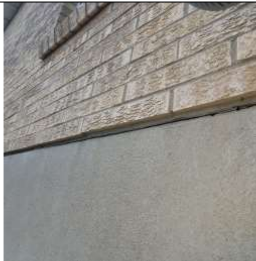
Wall/foundation black vapor barrier, asbestos
