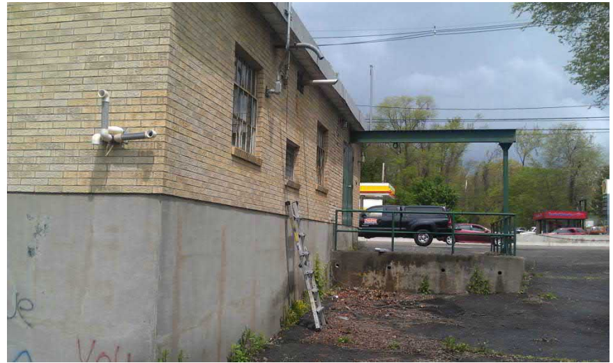
ACM – Window and Louvered Vent Caulking
