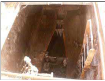
PHOTO 1 PARSHALL FLUME PR-3
