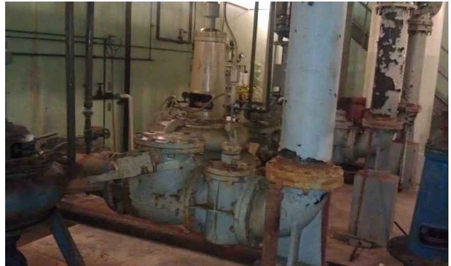
LBP on Basement Pump Equipment
