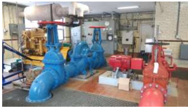
Interior – Main pump room
