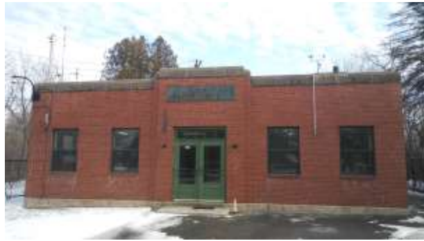
Exterior asbestos door and window caulk
