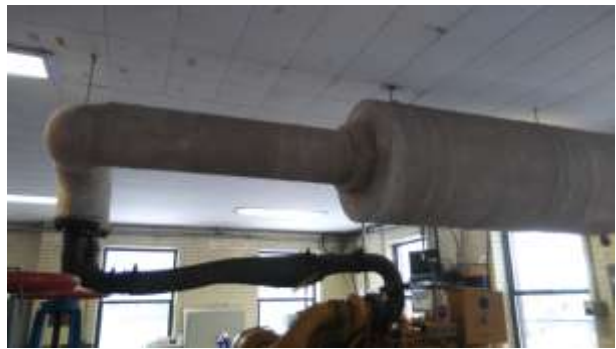
Non-asbestos generator exhaust insulation
