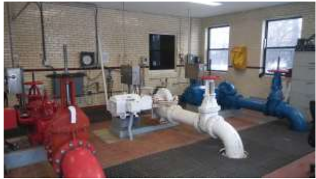
Interior – Main pump room
