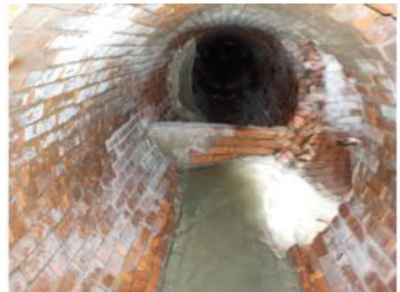
Photograph of OF-210: OF-211 pipe is to the right and brick weir is the regulator
