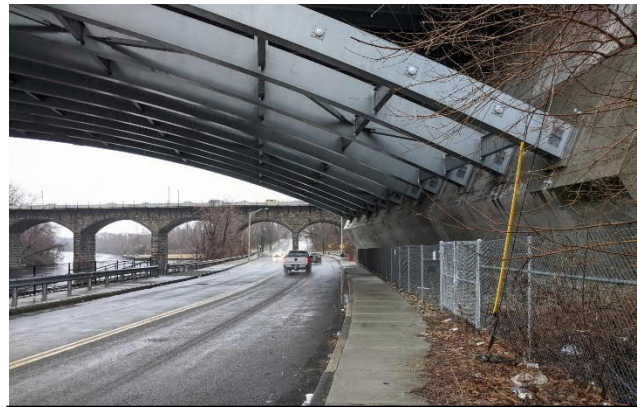
View of southbound lane of Taft Street beneath Route 95 Bridge looking towards the Division Street Bridge
