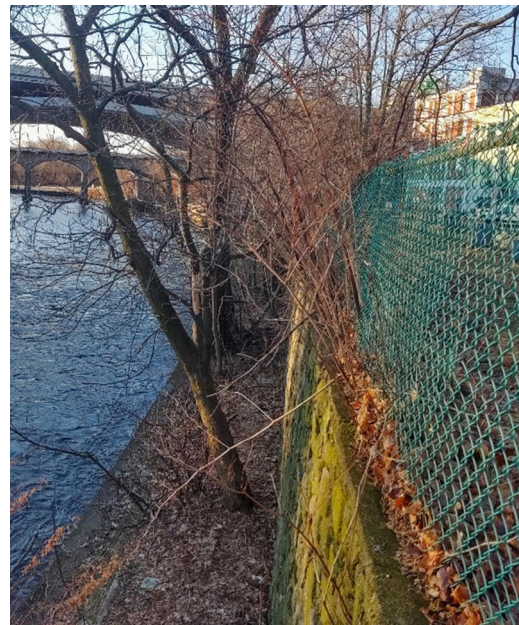
View of retaining wall - facing south, with the Seekonk River to the left and Taft Street to the right
