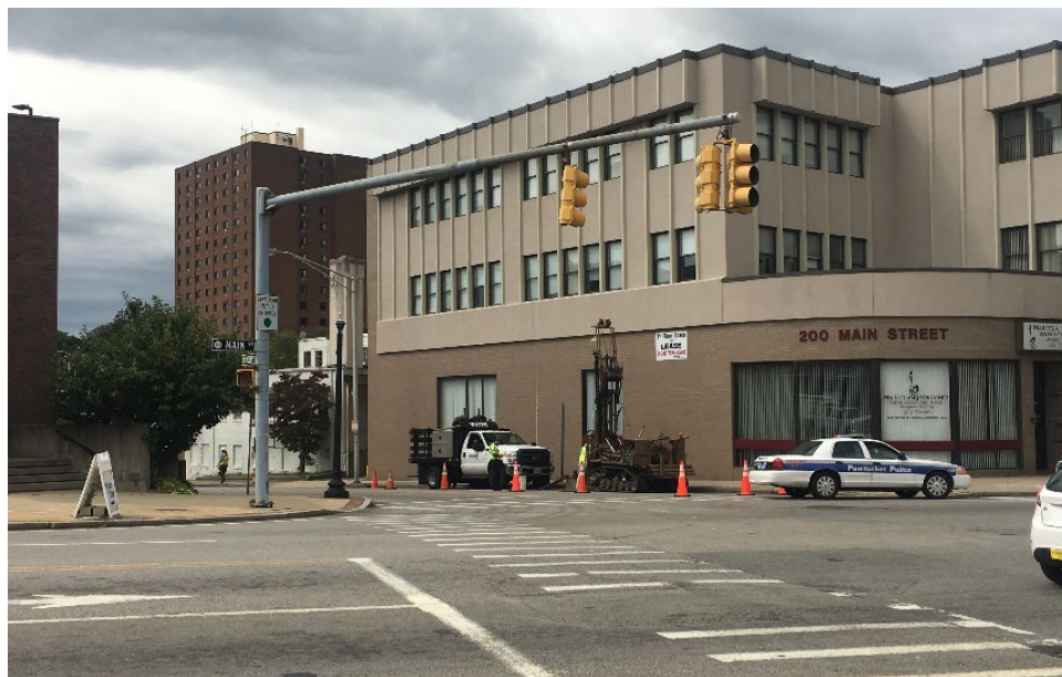
Drilling Test Boring B-8 at the Intersection of South Main St. and Roosevelt Ave. Ext.
