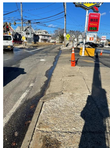
Image 1: Poor Sidewalk Conditions (East side of Elliot Street)
