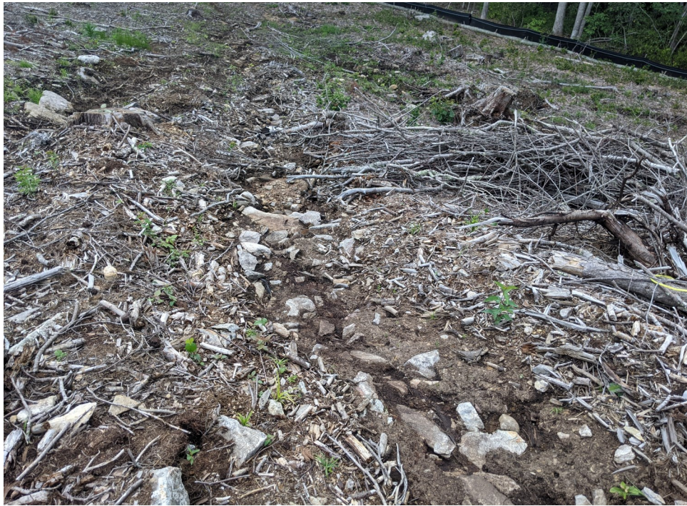
View erosion gullies beginning to form upgradient of the informal northern access road—facing northwest.
