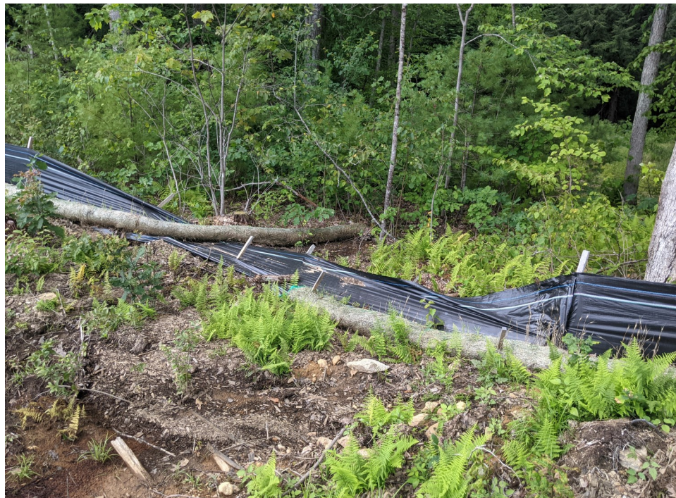
View of the erosion control breach—facing northwest.
