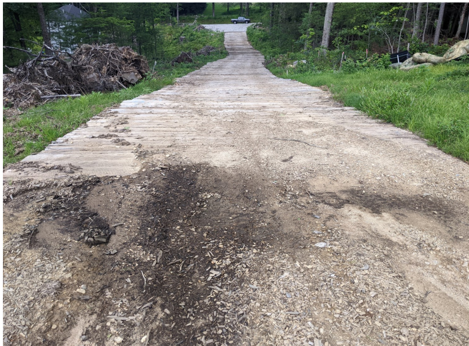
View of erosion within the access road to the north of the stockpile area—facing north.
