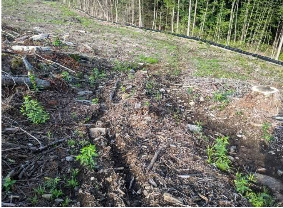
View of erosion channels and exposed soils within and along the equipment tracks present at the informal access road near the northern limits of work—facing northwest.
