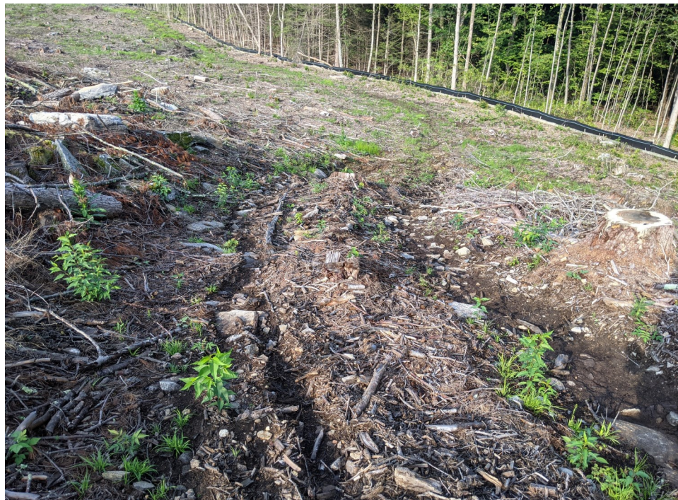
View of erosion gullies and exposed soils resulting from the informal access road along the northern limits of work—facing northwest.
