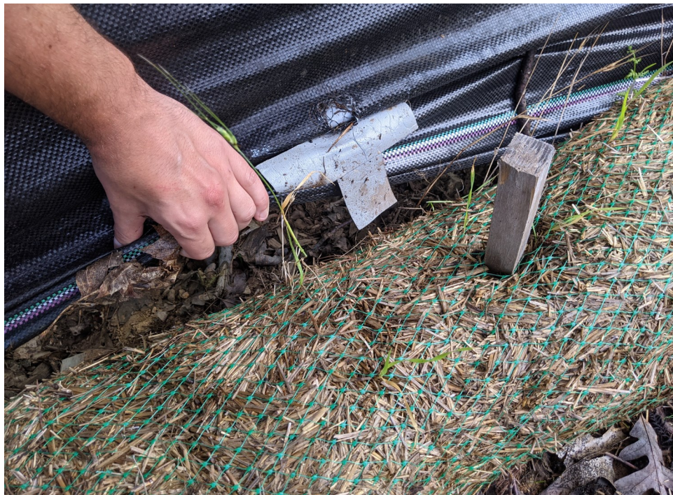
View of the siltation fencing incorrectly re-installed.
