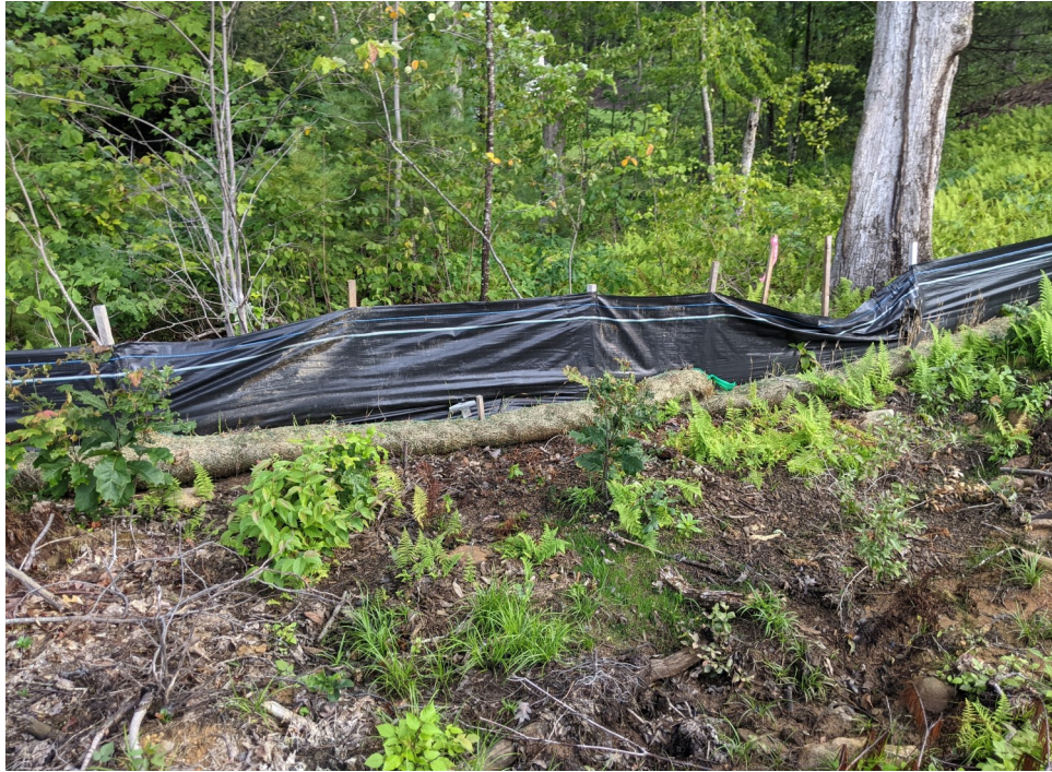
View of re-established straw wattles, rather than installation of a compost filter tube—facing north.
