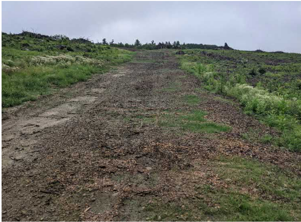
View of conditions within the access road leading to the stockpile area—facing south.
