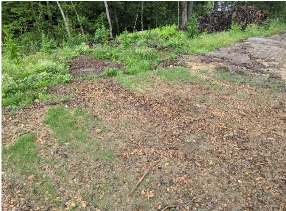
View of an area contributing runoff to the area of the former erosion control breach; note the channel forming to the left of the timber mats—facing northwest.
