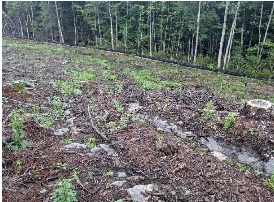
View of erosion channels and exposed soils within and along the equipment tracks present at the informal access road near the northern limits of work—facing northwest.
