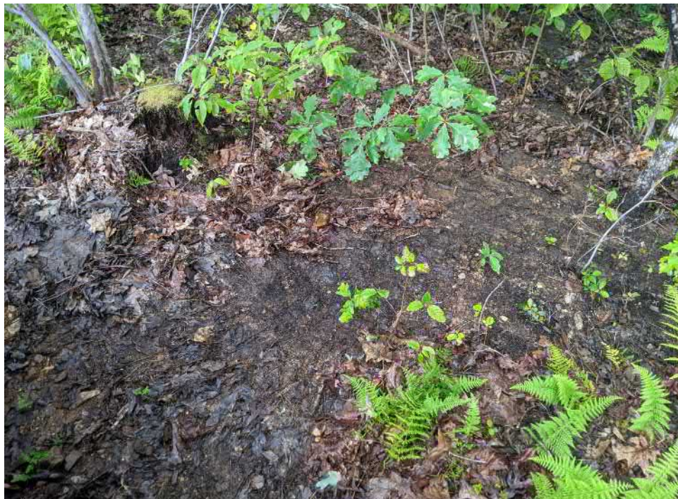
View of evidence that stormwater had flowed under the siltation fencing and discharged downgradient of the limits of work.
