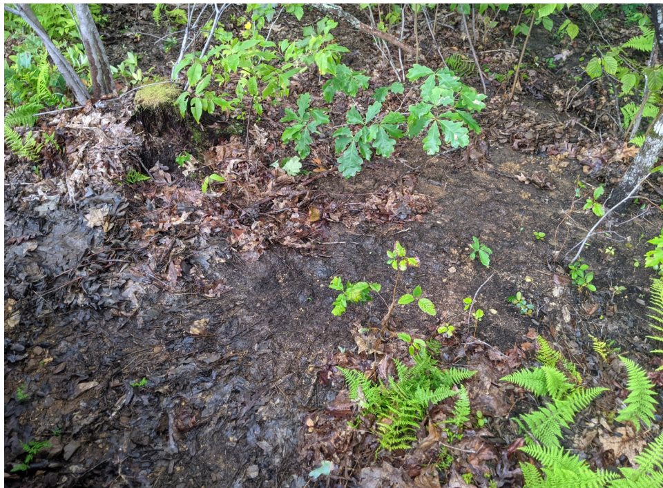
View of evidence that stormwater had flowed under the siltation fencing and discharged downgradient of the limits of work.
