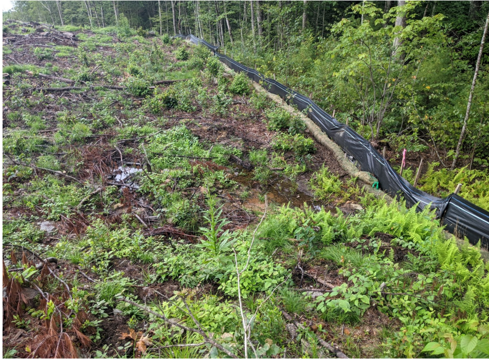
View of ponding water within the area of the former erosion control breach—facing north-west.
