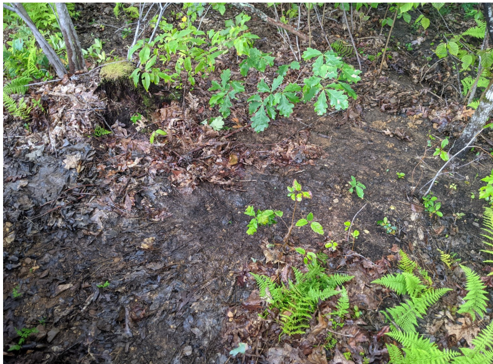
View of evidence of stormwater flowing under the siltation fencing and discharging downgradient of the limits of work.
