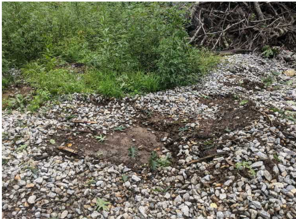
View of exposed soils along the west side of the stabilized construction entrance—facing west.
