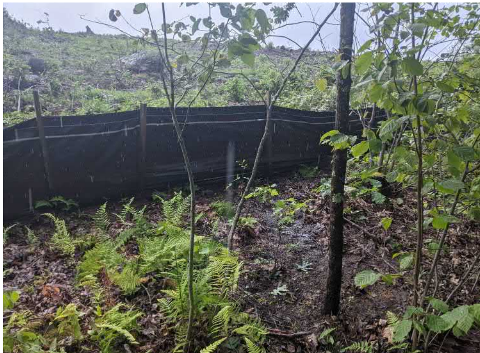
View of runoff undercutting the siltation fencing at the area of erosion controls that required maintenance as identified on 7/22/2021 - facing southwest.
