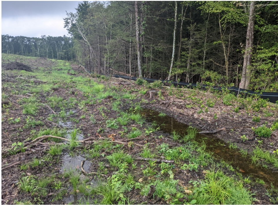
View of ponding associated with the runoff flowing down the access path depicted in Photo 6—facing northwest.
