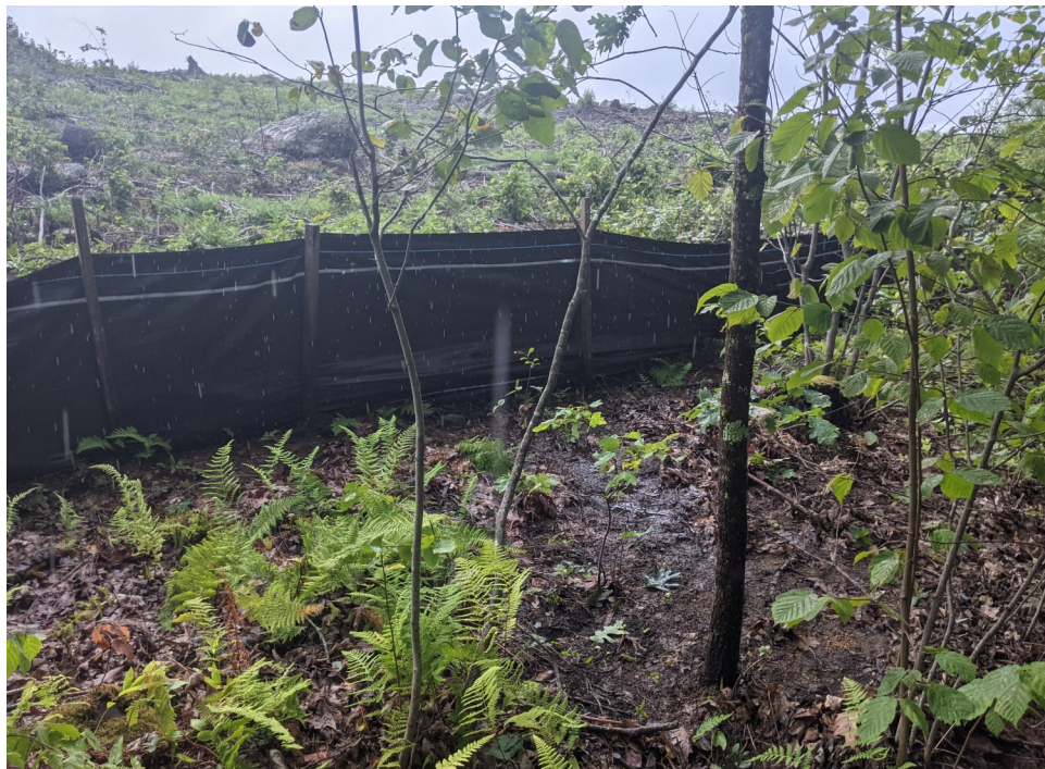
View of runoff undercutting the siltation fencing at the area of erosion controls that required maintenance as identified on 7/22/2021 - facing southwest.
