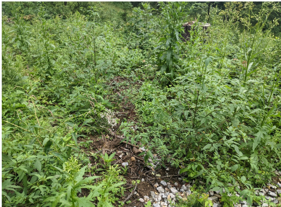
View of scour associated with the exposed soils at the construction entrance; this scour is confined to the limits of work—facing southwest.
