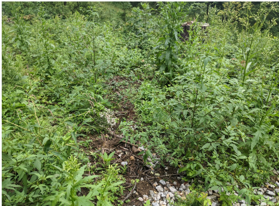
View of scour associated with the aforementioned exposed soils at the construction entrance; all scour is confined to the limits of work—facing southwest.
