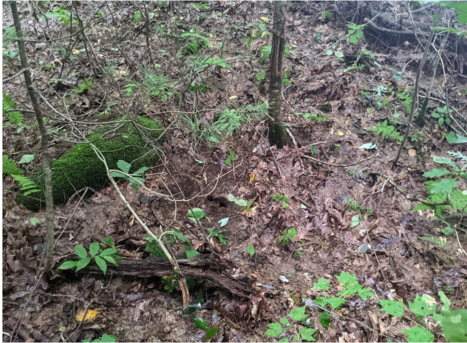
View of scour forming just upgradient of the off-site Vegetated Wetland—facing east.
