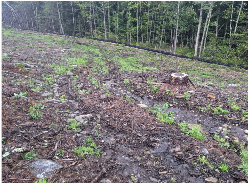
View of erosion channels at the location of the informal access path along the northern limits of work—facing northwest.
