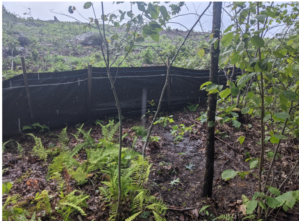
View of runoff undercutting the siltation fencing at the location of the former erosion control breach (Discharge 1) - facing southwest.
