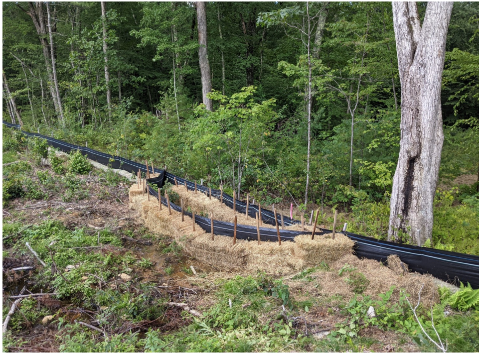
View of the repaired erosion control measures associated with Discharge 1—facing north-west.
