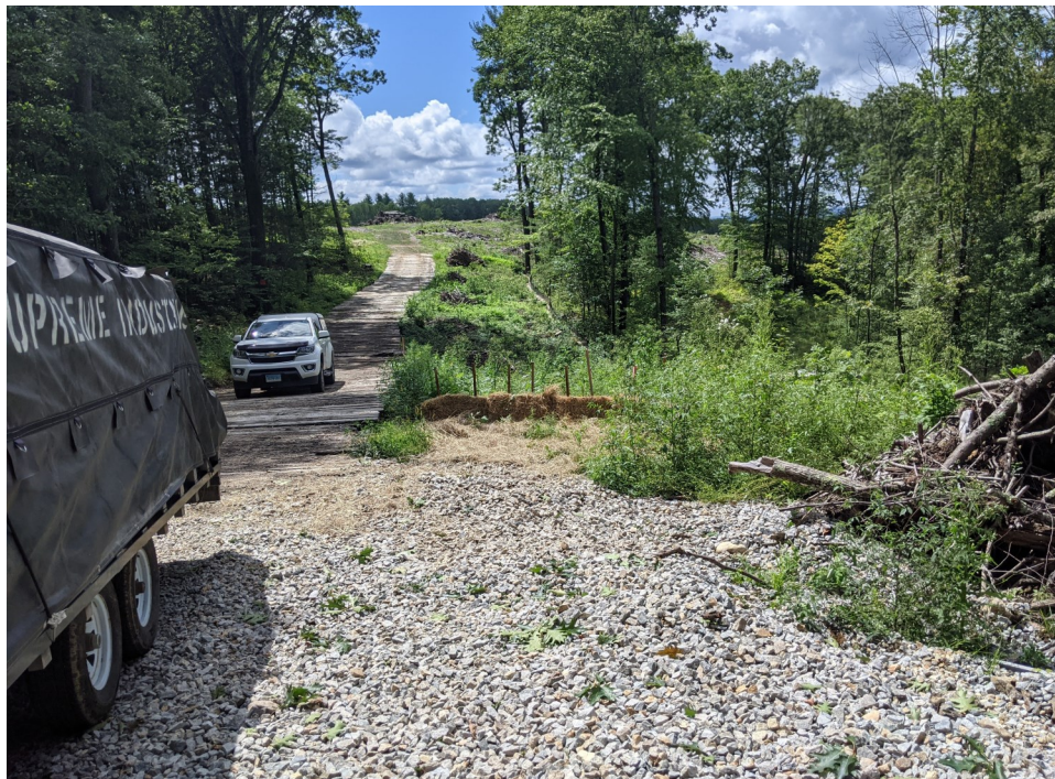
View of exposed soils stabilized at the construction entrance; note the implementation of straw bales—facing south.
