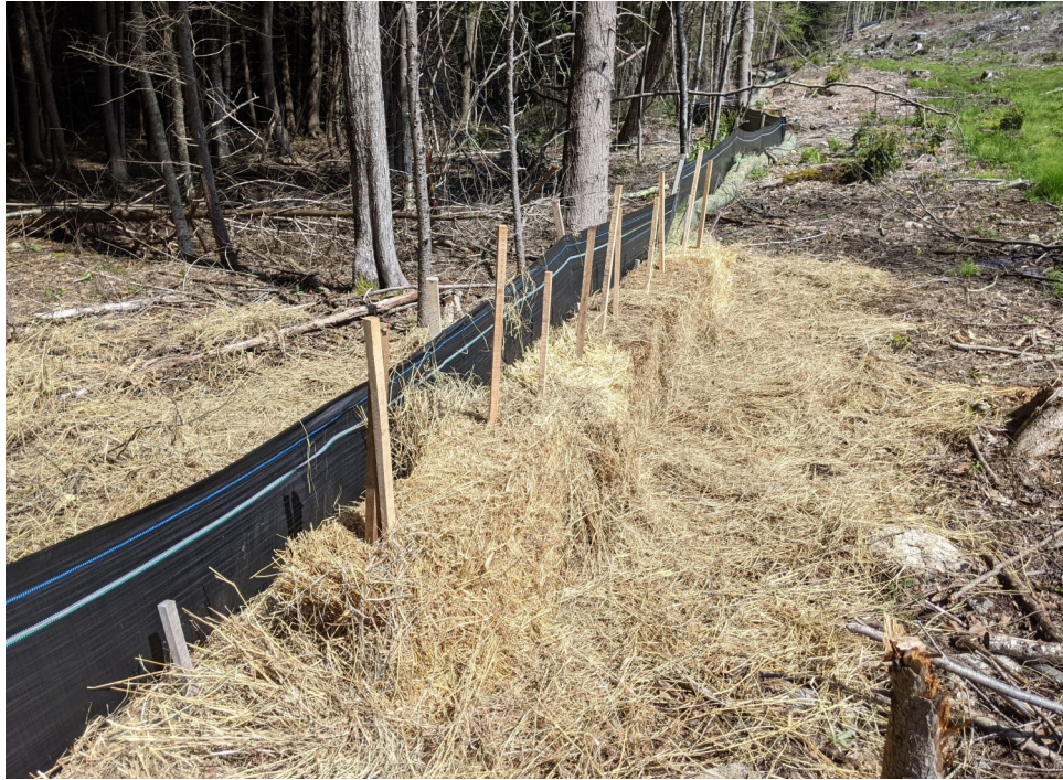
View of the repaired erosion control breach associated with Discharge 2; note the stabilization of exposed soils beyond the limits of work—facing northeast.
