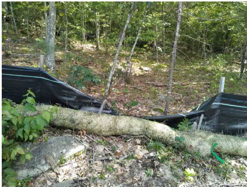
View of the damaged silt fence in southern perimeter of Site —facing south.
