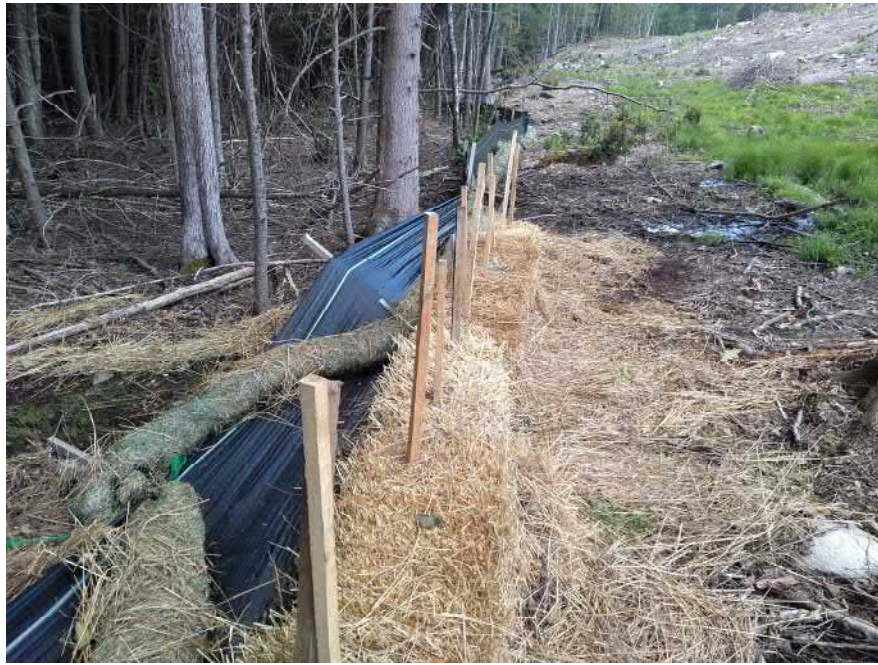
View of the damage erosion control measures associated with Discharge 2—facing north.
