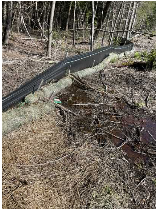
View of the damage erosion control measures associated with Discharge 2—facing north.
