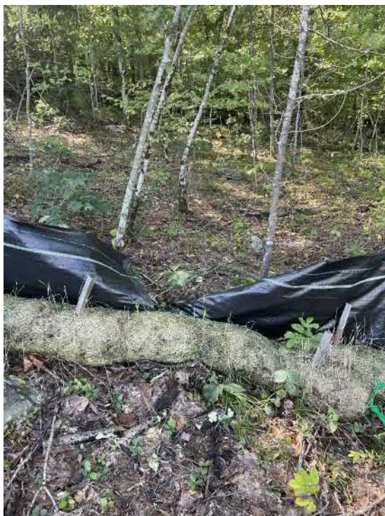
View of the damaged silt fence in southern perimeter of Site —facing south.
