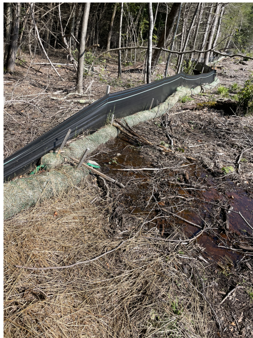
View of degraded straw wattle at southeast perimeter of Site —facing east.
