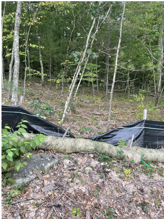
View of the damaged silt fence in southern perimeter of Site —facing south.
