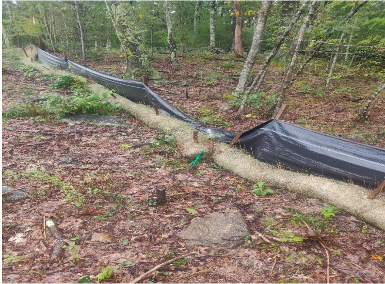
View of the damaged silt fence in southern perimeter of Site —facing south.
