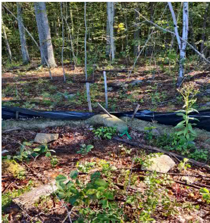
View of damaged silt fence in south east portion of the Site —facing south east
