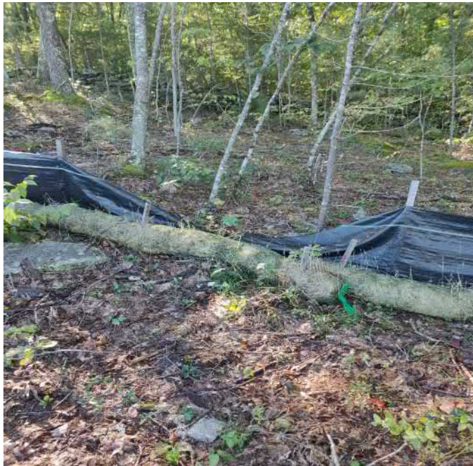
View of the damaged silt fence in southern perimeter of Site —facing south.
