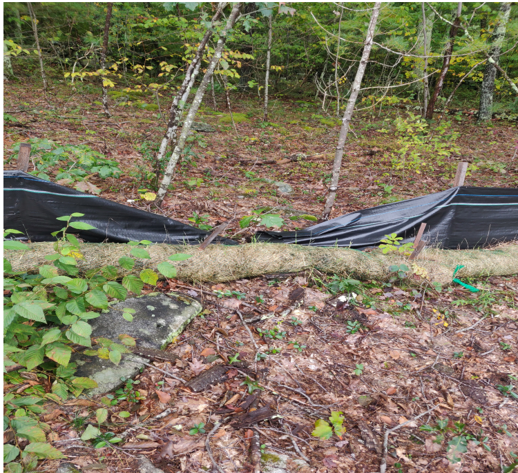
View of damaged silt fence in south east portion of the Site —facing south east
