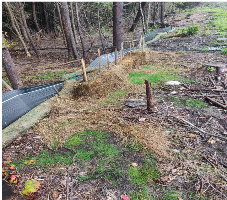
View of area downgradient of Discharge 2—facing north west.
