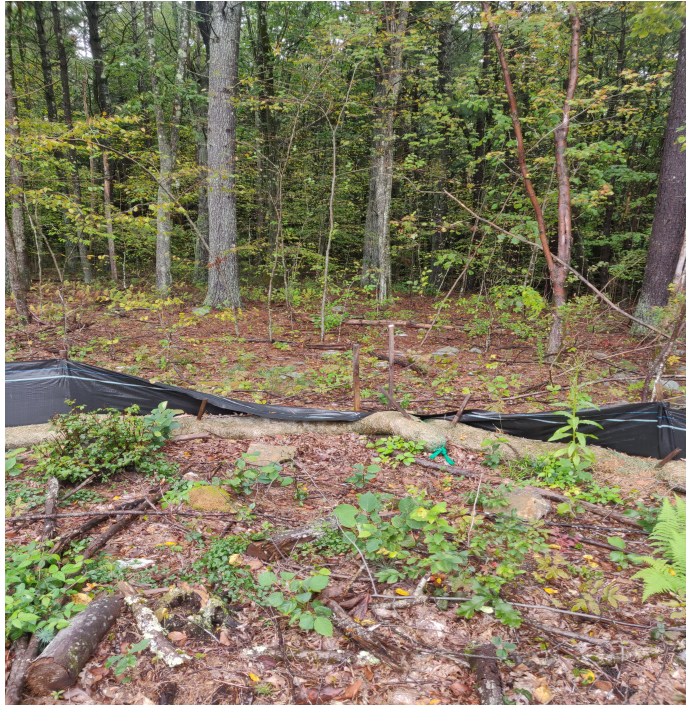
View of the damaged silt fence in southern perimeter of Site —facing south.
