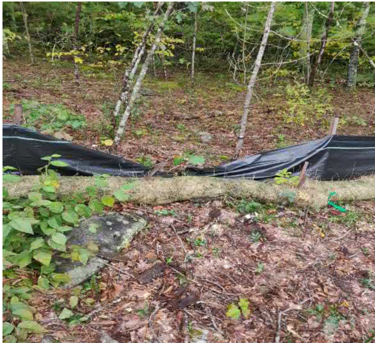
View of damaged silt fence in south east portion of the Site —facing south east
