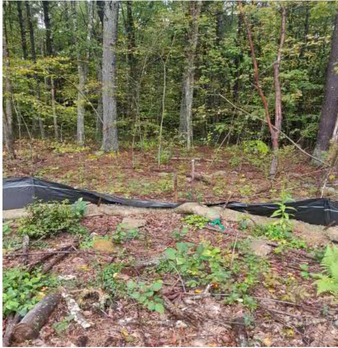
View of the damaged silt fence in southern perimeter of Site —facing south.
