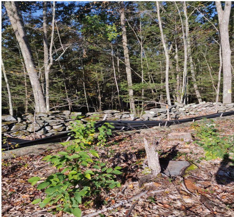
View of damaged silt fence in south west portion of the Site —facing south west
