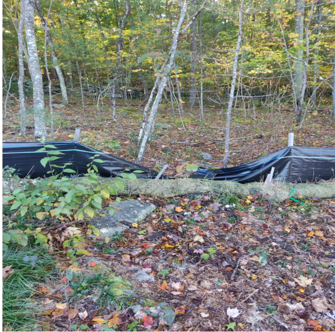
View of the damaged silt fence in southern perimeter of Site —facing south.
