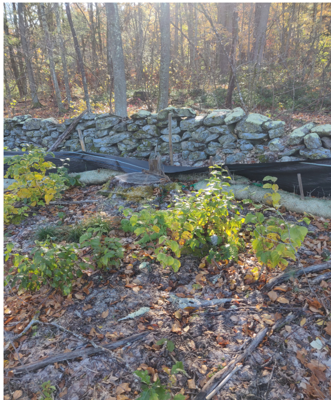
View of damaged silt fence in eastern portion of the Site —facing east
