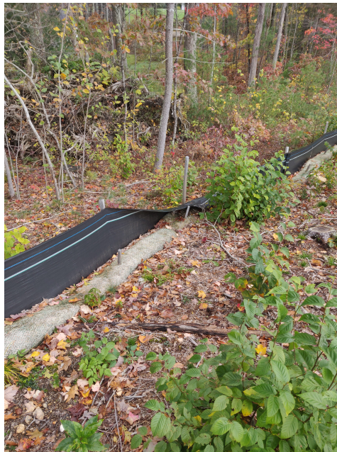
View of damaged silt fence in north western portion of the Site —facing north west
