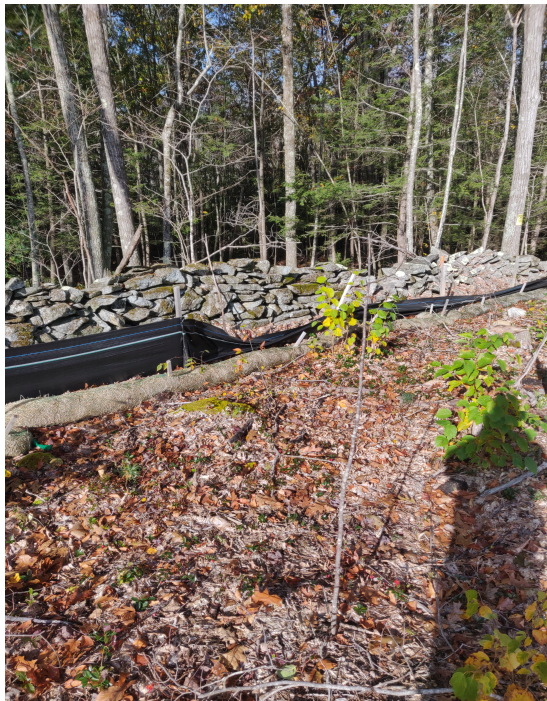
View of damaged silt fence in south west portion of the Site —facing south west
