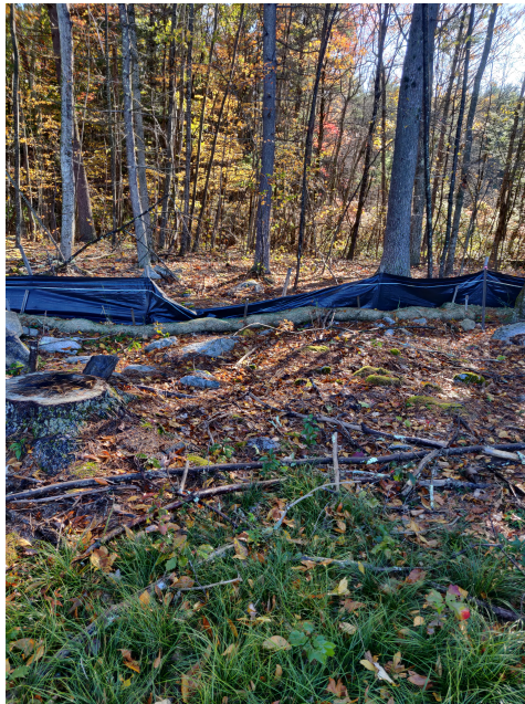
View of damaged silt fence in eastern portion of the Site —facing east
