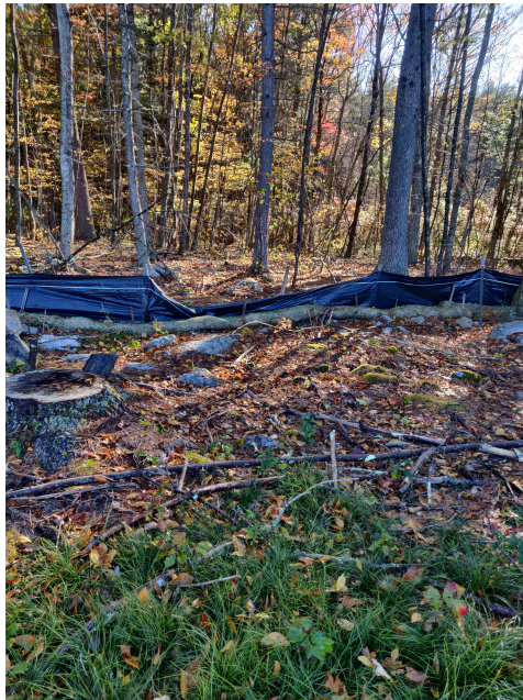
View of damaged silt fence in eastern portion of the Site —facing east
