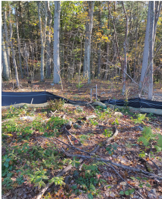
View of damaged silt fence in south east portion of the Site —facing south east
