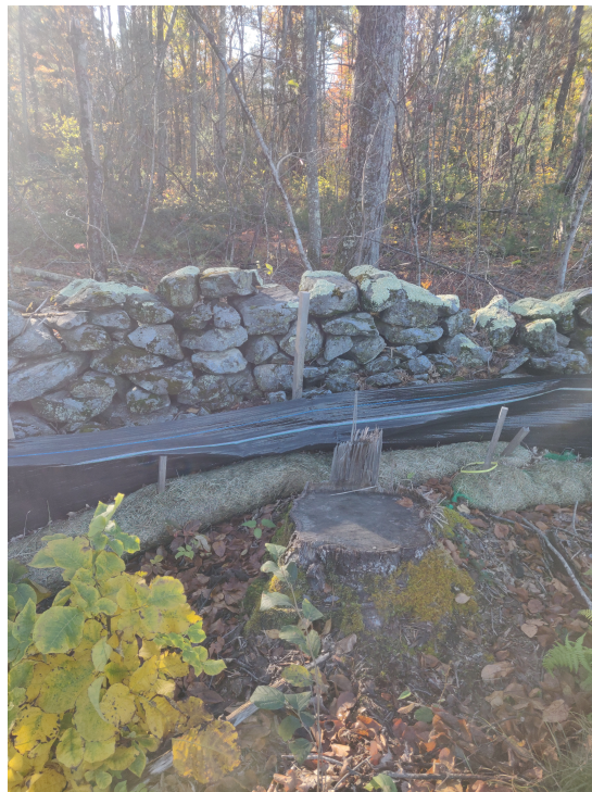
View of damaged silt fence in eastern portion of the Site —facing east
