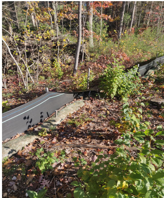
View of damaged silt fence in north western portion of the Site —facing north west
