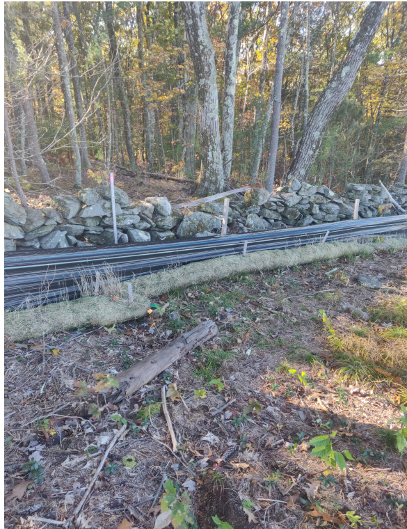
View of damaged silt fence in eastern portion of the Site —facing east
