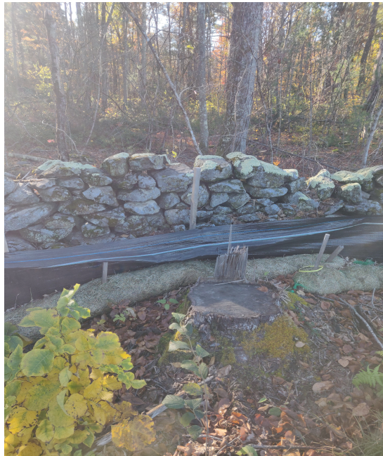
View of damaged silt fence in south west portion of the Site —facing south west
