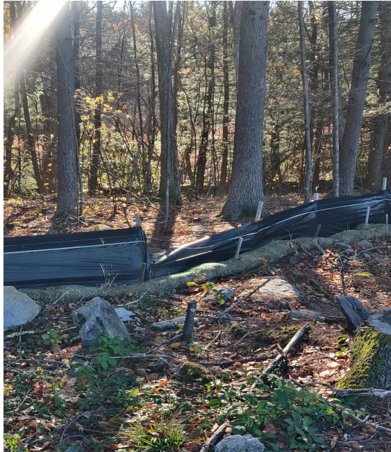
View of damaged silt fence in eastern portion of the Site —facing east
