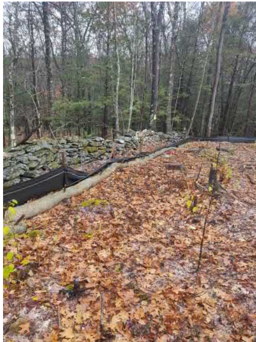
View of damaged silt fence in south west portion of the Site —facing south west
