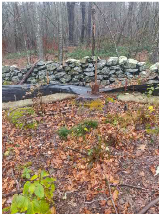
View of damaged silt fence in south west portion of the Site —facing south west
