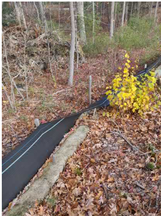
View of damaged silt fence in north western portion of the Site —facing north west
