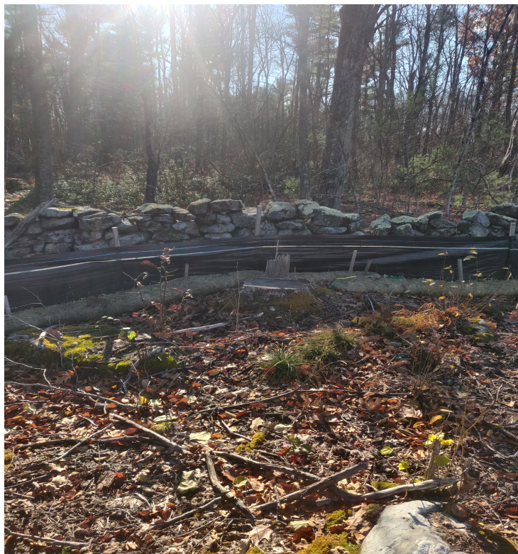
View of damaged silt fence in eastern portion of the Site —facing east
