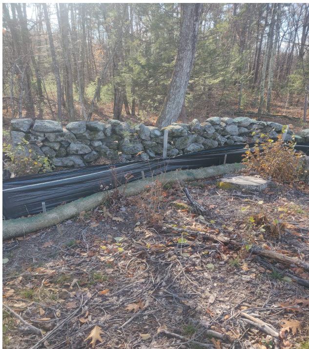
View of damaged silt fence in south west portion of the Site —facing south west
