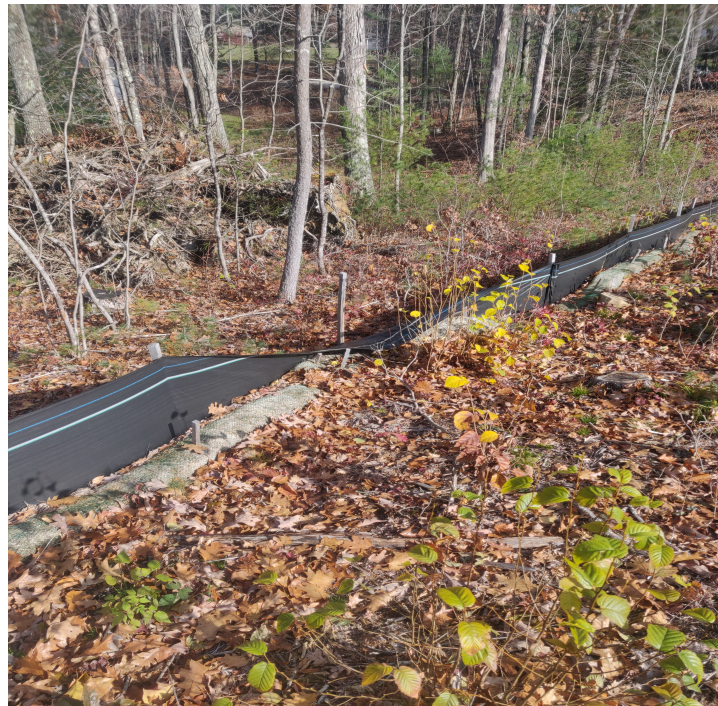
View of damaged silt fence in north western portion of the Site —facing north west
