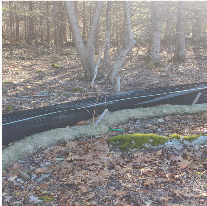
View of damaged silt fence in eastern portion of the Site —facing east
