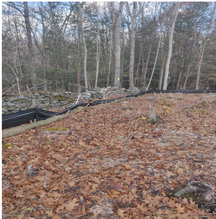
View of damaged silt fence in south west portion of the Site —facing south west
