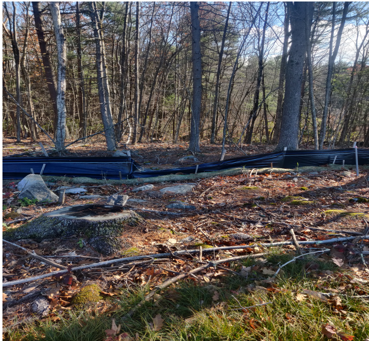
View of damaged silt fence in eastern portion of the Site —facing east
