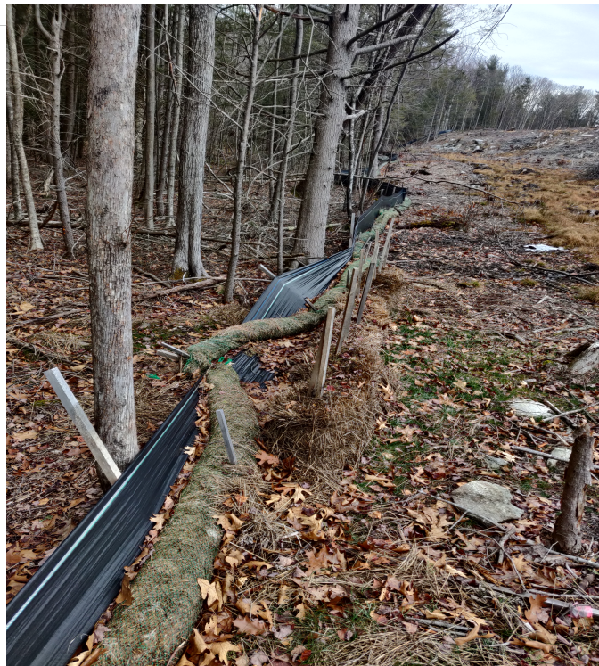
View of area downgradient of Discharge 2—facing north west.
