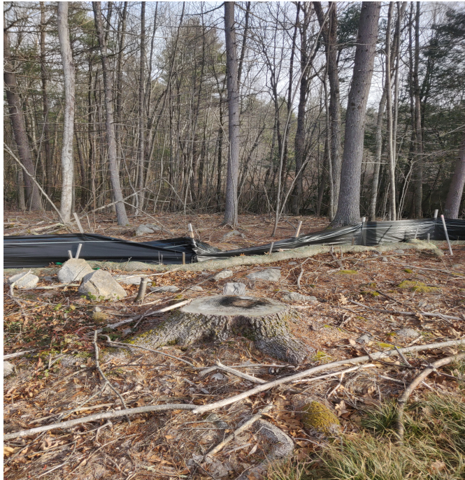
View of damaged silt fence in eastern portion of the Site —facing east
