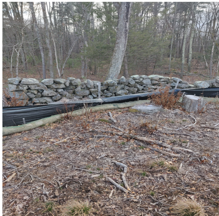
View of damaged silt fence in south west portion of the Site —facing south west
