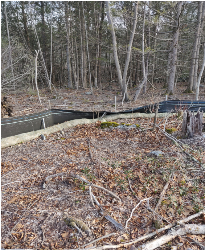
View of damaged silt fence in eastern portion of the Site —facing east
