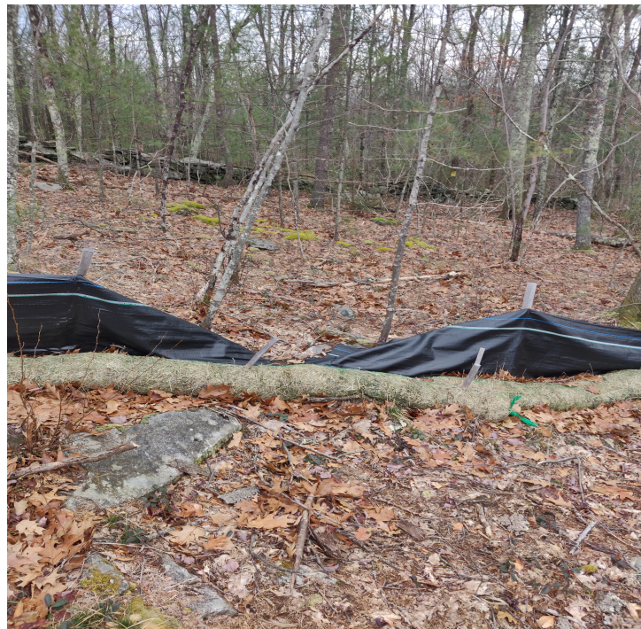
View of damaged silt fence in south east portion of the Site —facing south east
