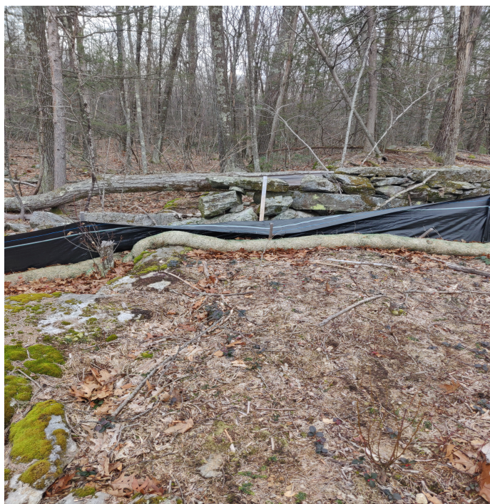
View of damaged silt fence and wattle in south eastern portion of the Site —facing south east
