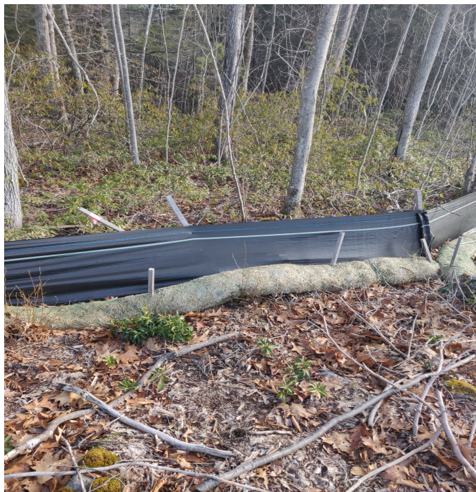
View of damaged silt fence and wattle in eastern portion of the Site —facing north east
