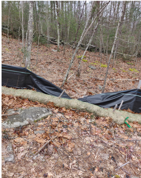
View of damaged silt fence in south east portion of the Site —facing south east
