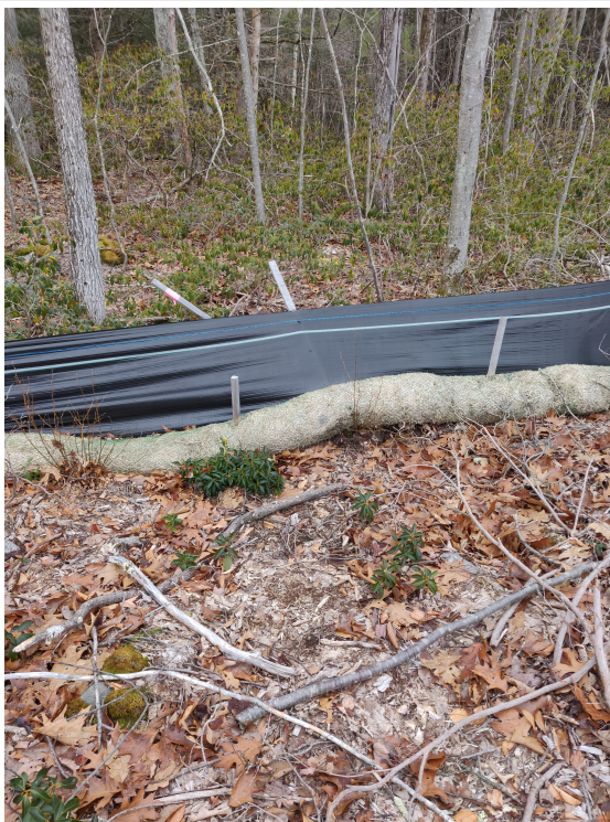
View of damaged silt fence and waddle in eastern portion of the Site —facing north east
