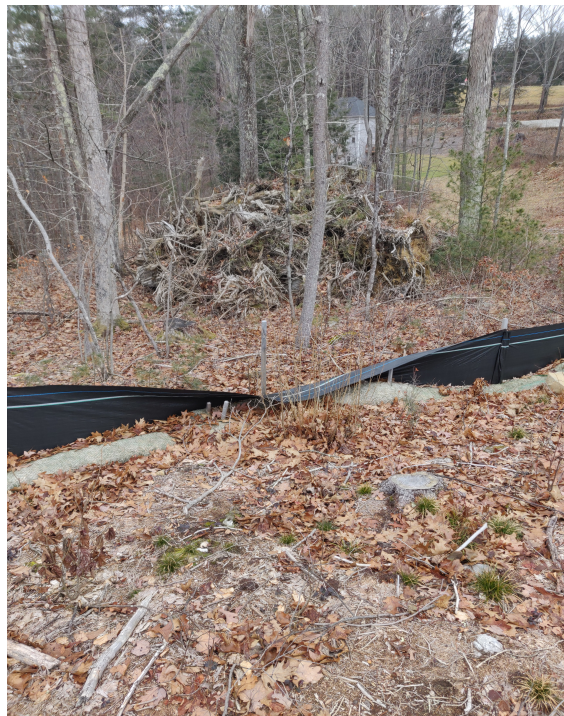
View of damaged silt fence in north western portion of the Site —facing north west
