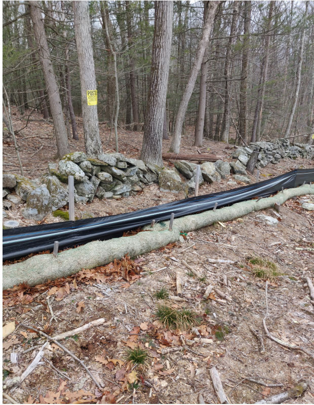
View of the damaged silt fence in eastern portion of Site — facing south east.
