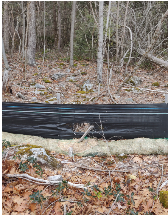
View of damaged silt fence and waddle in eastern portion of the Site —facing east
