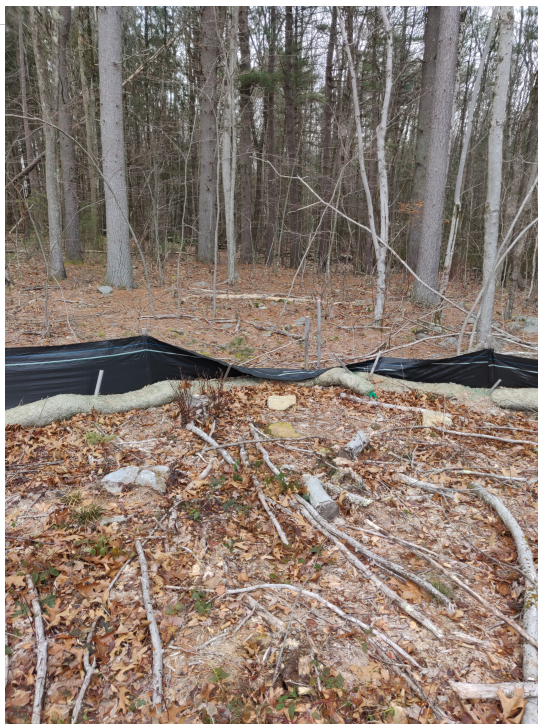
View of damaged silt fence and waddle in south eastern portion of the Site —facing south east
