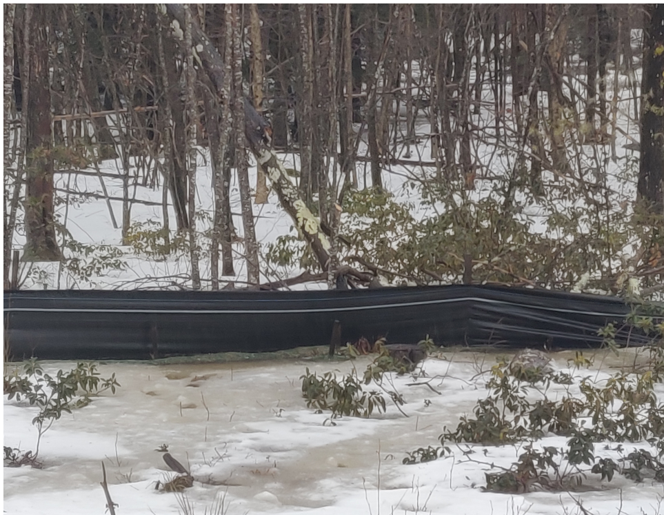
View of the flooded straw wattle and silt fence located up-gradient from Discharge 2 — Facing north west
