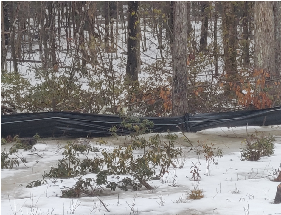
Photo 4 View of the flooded straw wattle and silt fence located up-gradient from Discharge 2 — Facing north west
