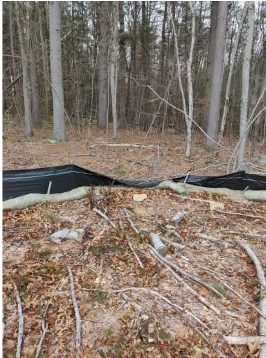
View of damaged silt fence and waddle in south eastern portion of the Site —facing south east
