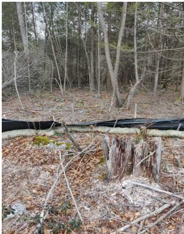
View of damaged silt fence in eastern portion of the Site —facing east
