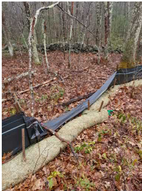
View of damaged silt fence in south east portion of the Site —facing south east
