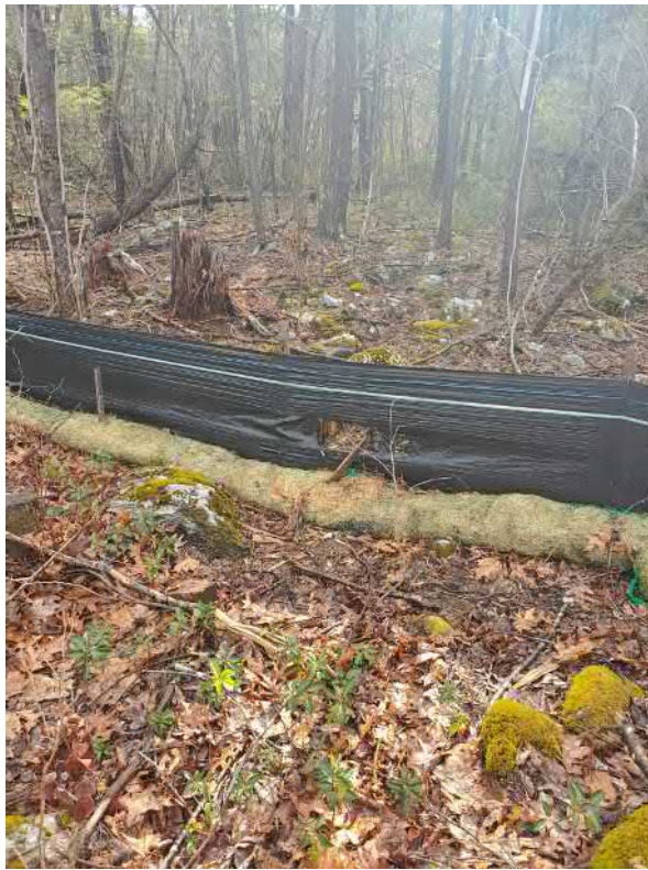
View of damaged silt fence in north east portion of the Site —facing north east
