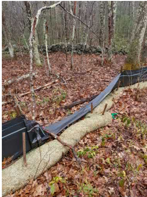
View of damaged silt fence in south east portion of the Site —facing south east
