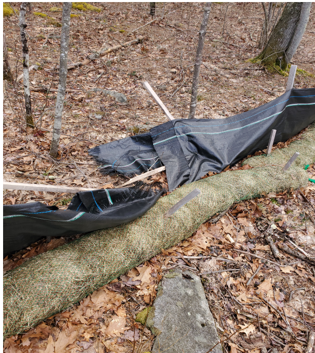
View of damaged silt fence in southeast portion of the Site —facing southeast
