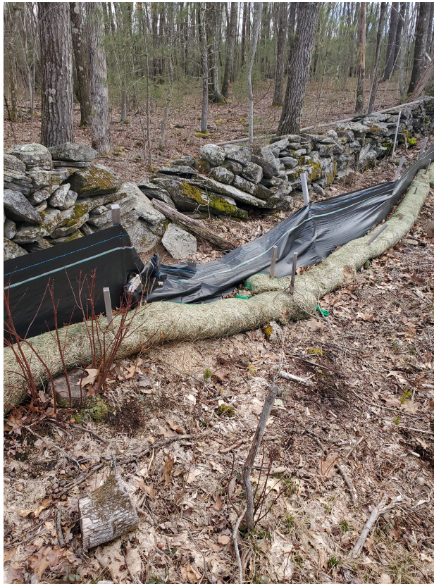
View of damaged silt fence in eastern portion of the Site —facing southeast
