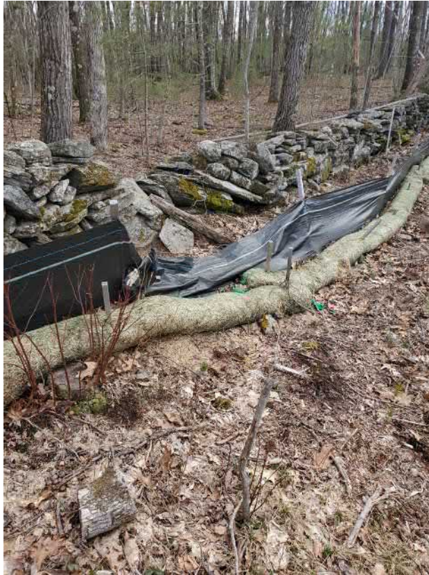
View of damaged silt fence in eastern portion of the Site —facing south
