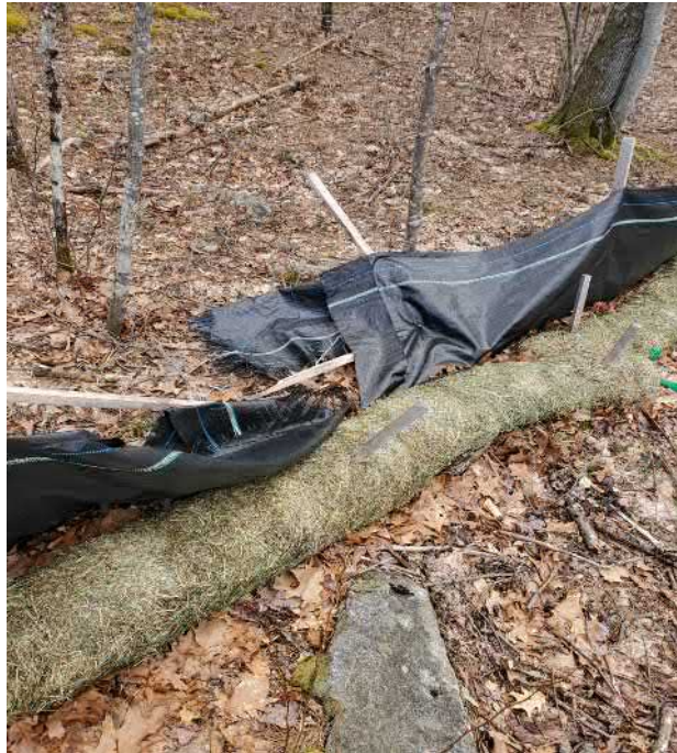
View of damaged silt fence in southern portion of the Site —facing south
