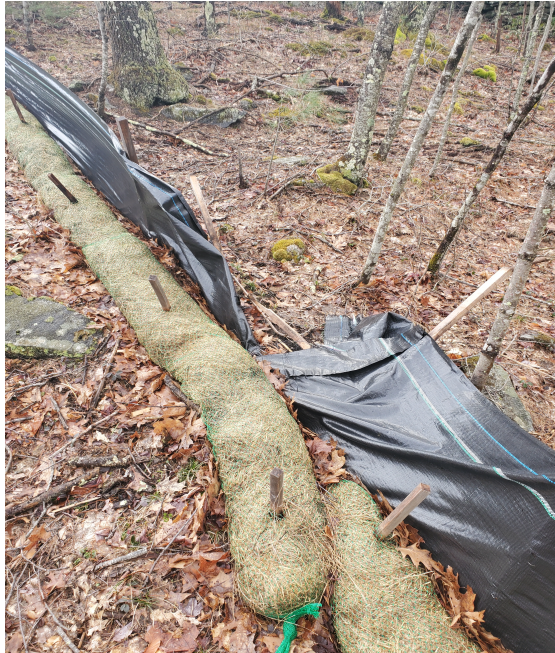
View of damaged silt fence in south east portion of the Site —facing south east
