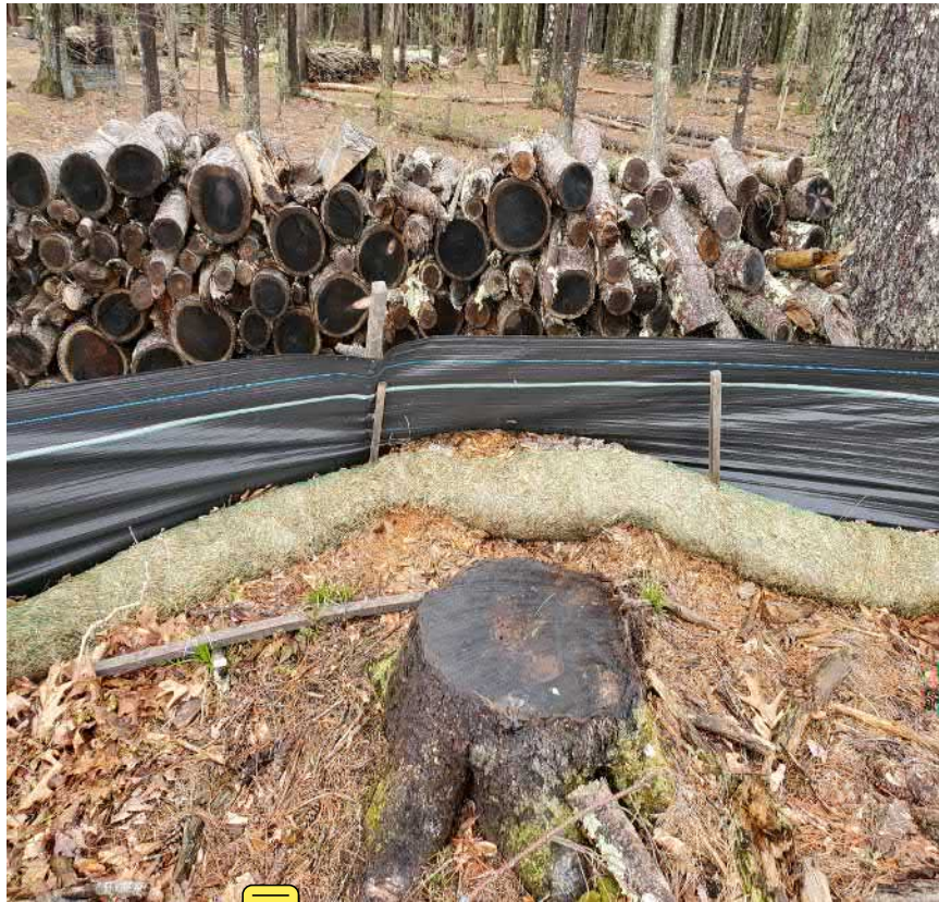
View of damaged silt wattle in northern portion of the Site —facing north
