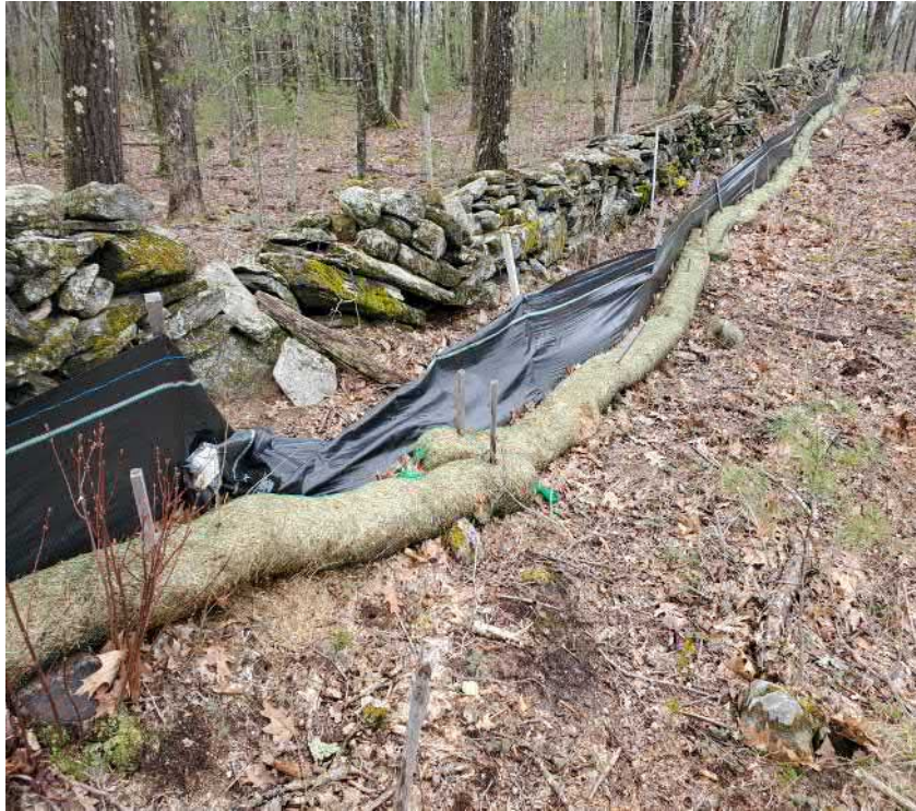
View of damaged silt fence in eastern portion of the Site —facing south east
