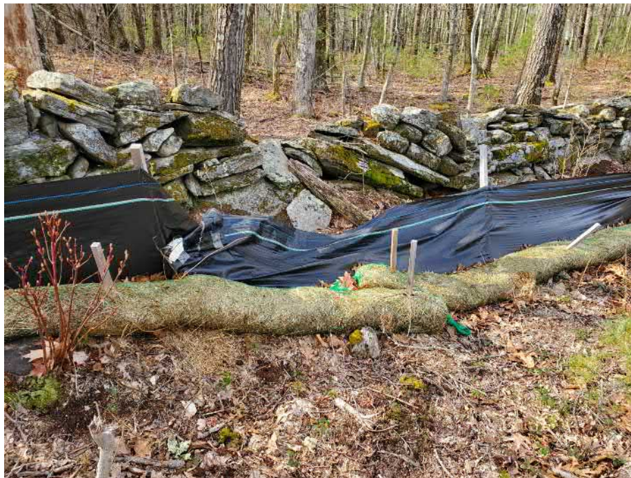
View of damaged silt fence in eastern portion of the Site — facing southeast
