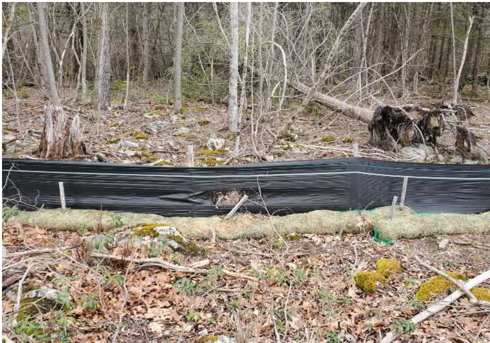
View of damaged silt wattle in northeastern portion of the Site — facing northeast
