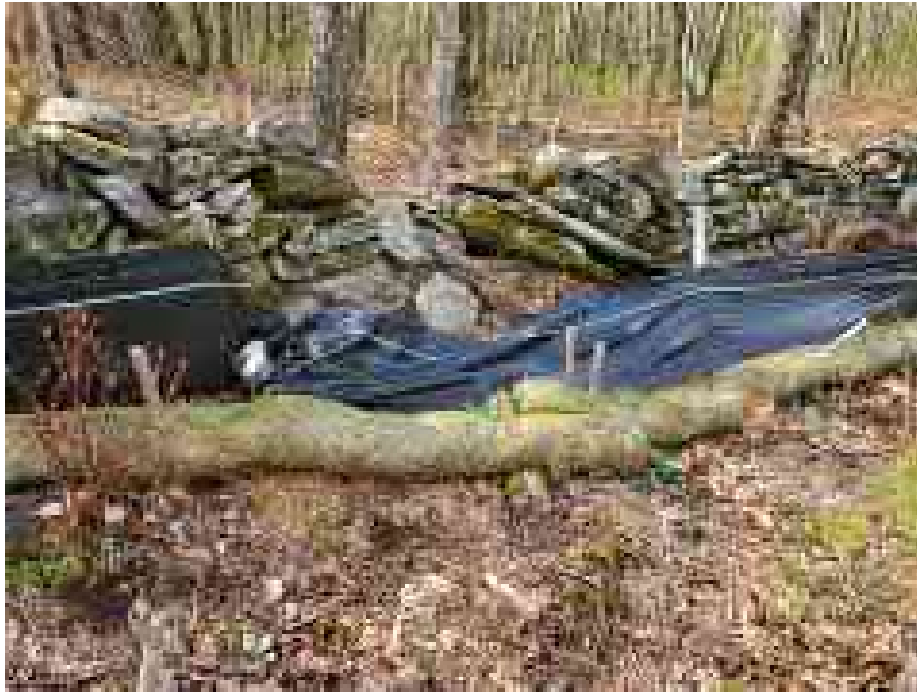
View of damaged silt fence in eastern portion of the Site — facing south east
