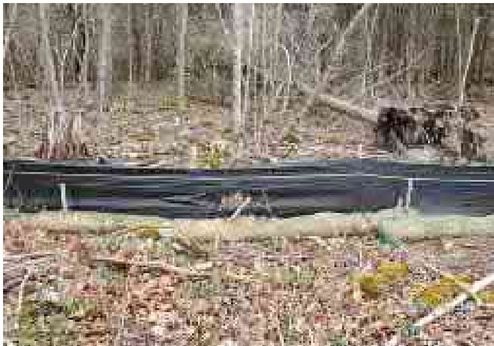
View of damaged silt wattle in northern portion of the Site — facing north east
