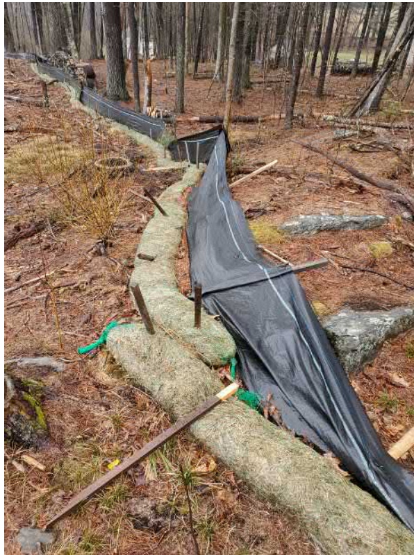
View of damaged silt fence in northern portion of the Site—facing north west.
