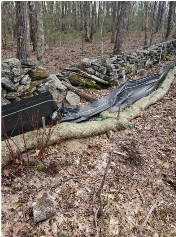
View of damaged silt fence in eastern portion of the Site —facing south east
