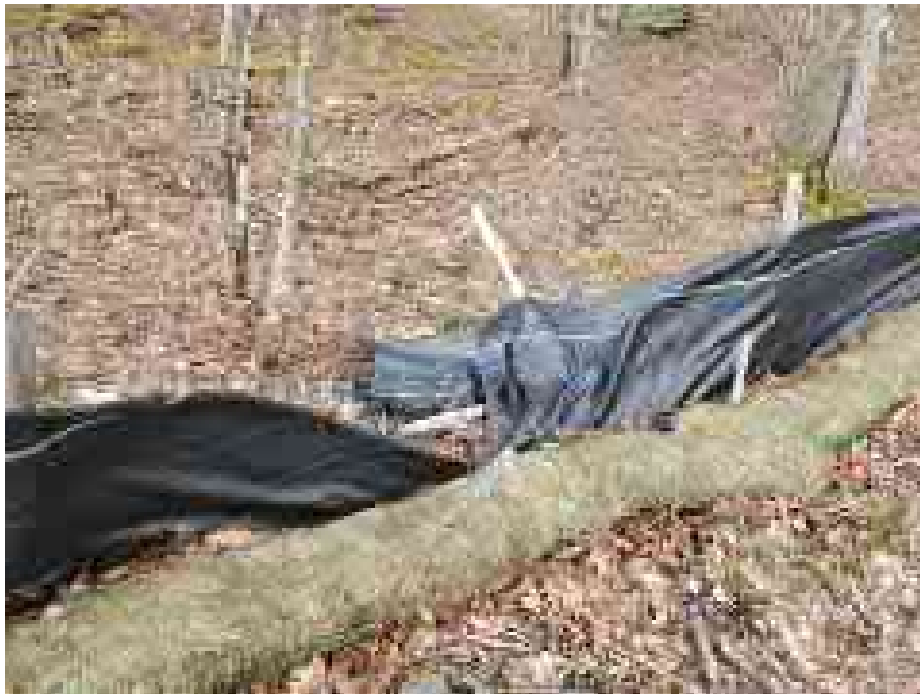
View of damaged silt fence in southern portion of the Site — facing south, east
