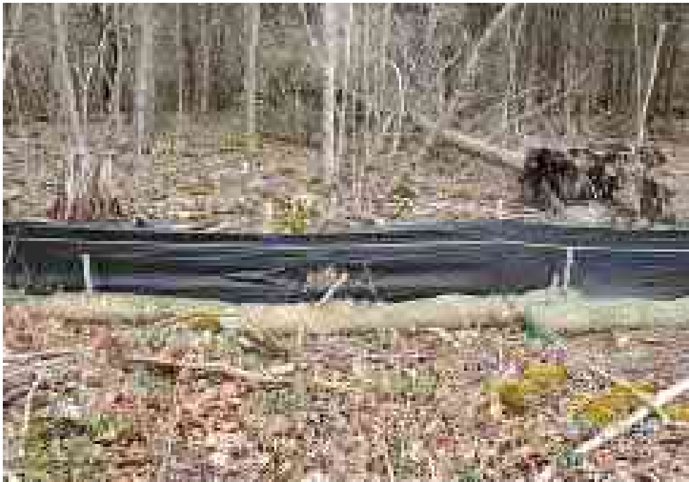
View of damaged silt wattle in northern portion of the Site — facing north
