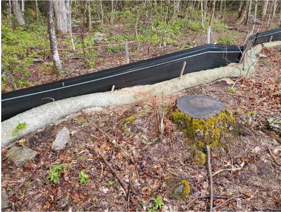
View of damaged silt wattle in northern portion of the Site — facing north
